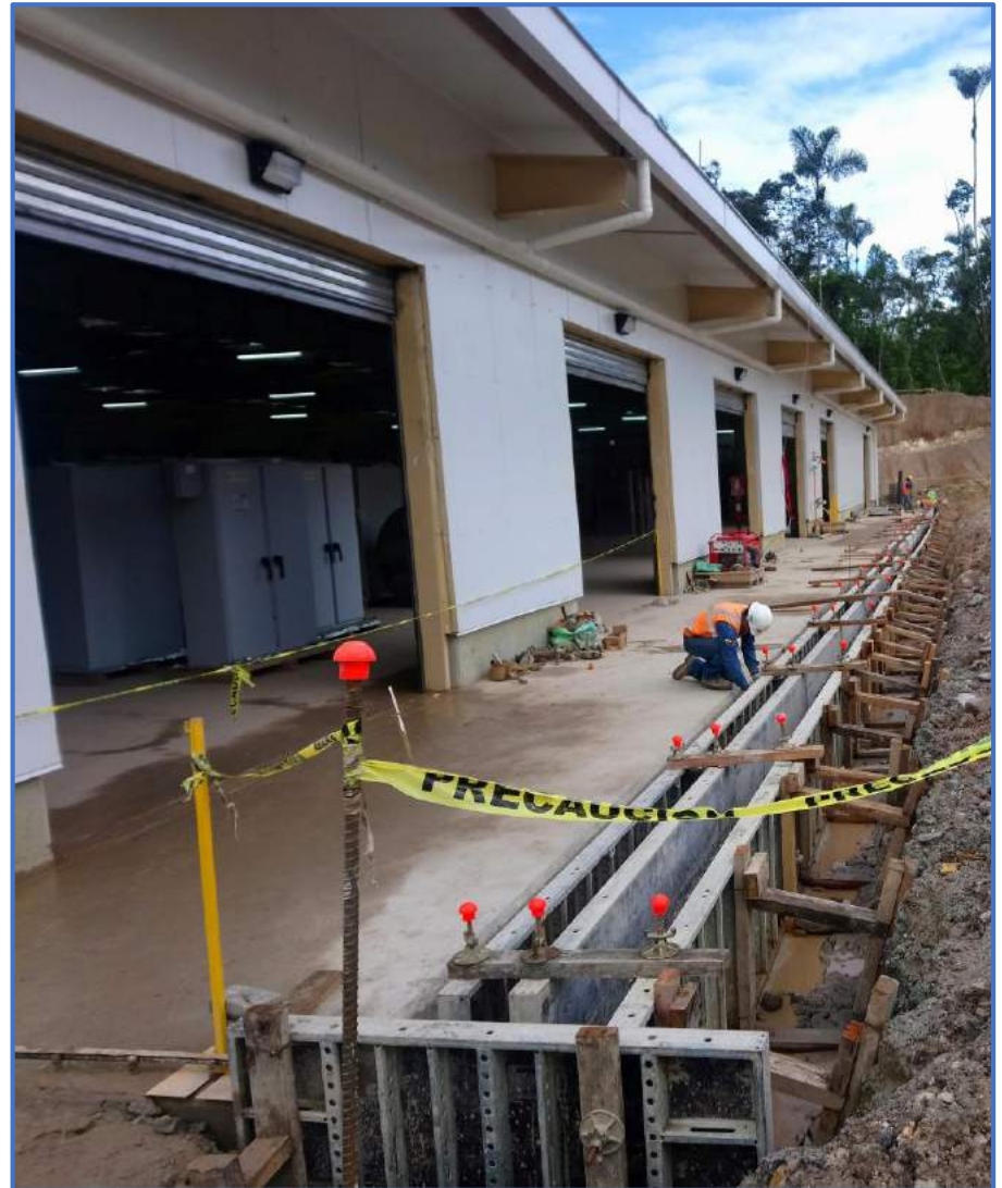
Reagent storage building
